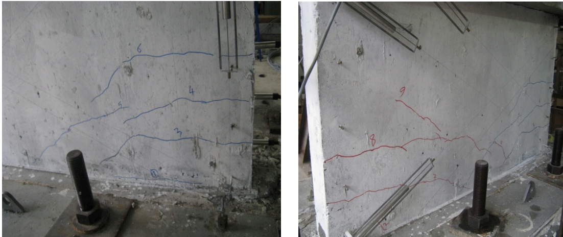
Figure 3.13. Initial Diagonal Cracks (T3-S1).
