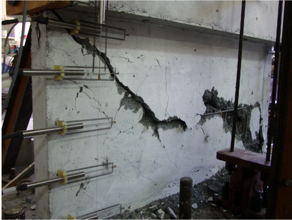
Figure 3.29. High Damage Level (T1-N10-S1).
