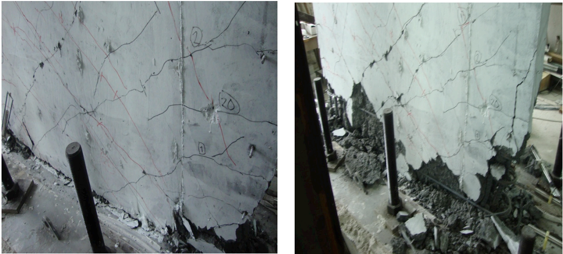
Figure 3.21. Medium and High Damage Levels (T5-S1).
