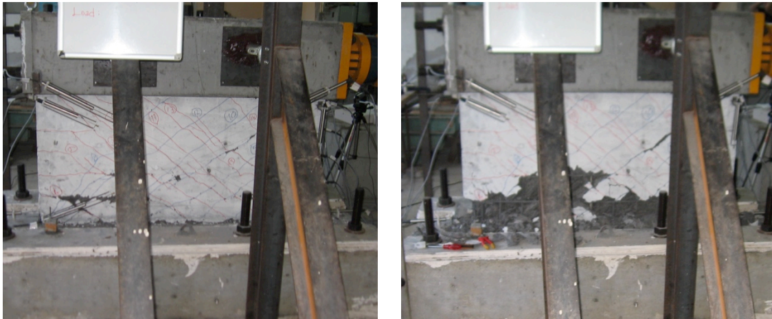
Figure 3.12. Medium and High Damage Levels (T2-S3).
