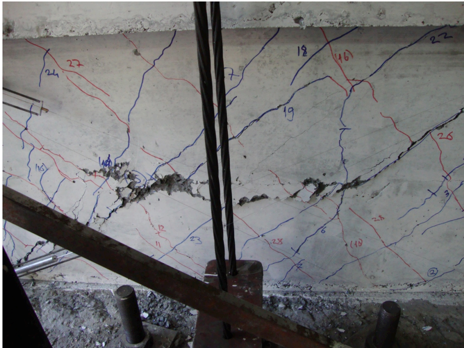
Figure 3.28. Main Crack (T1-N10-S1).
