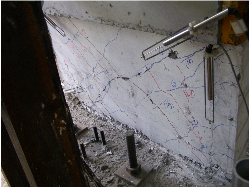
Figure 3.25. Main Diagonal Crack at Ultimate Load (T1-S2).
