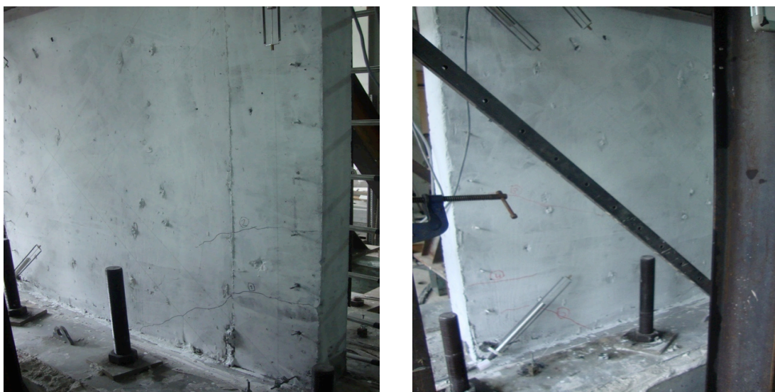
Figure 3.19. Initial Diagonal Cracks (T5-S1).
